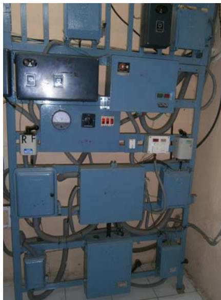
Fig. 4.14 Electrical control panel
